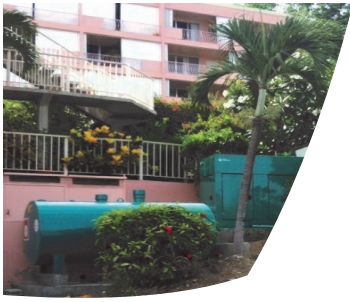
WORKING Generator at the West End of H-Building !!!!
